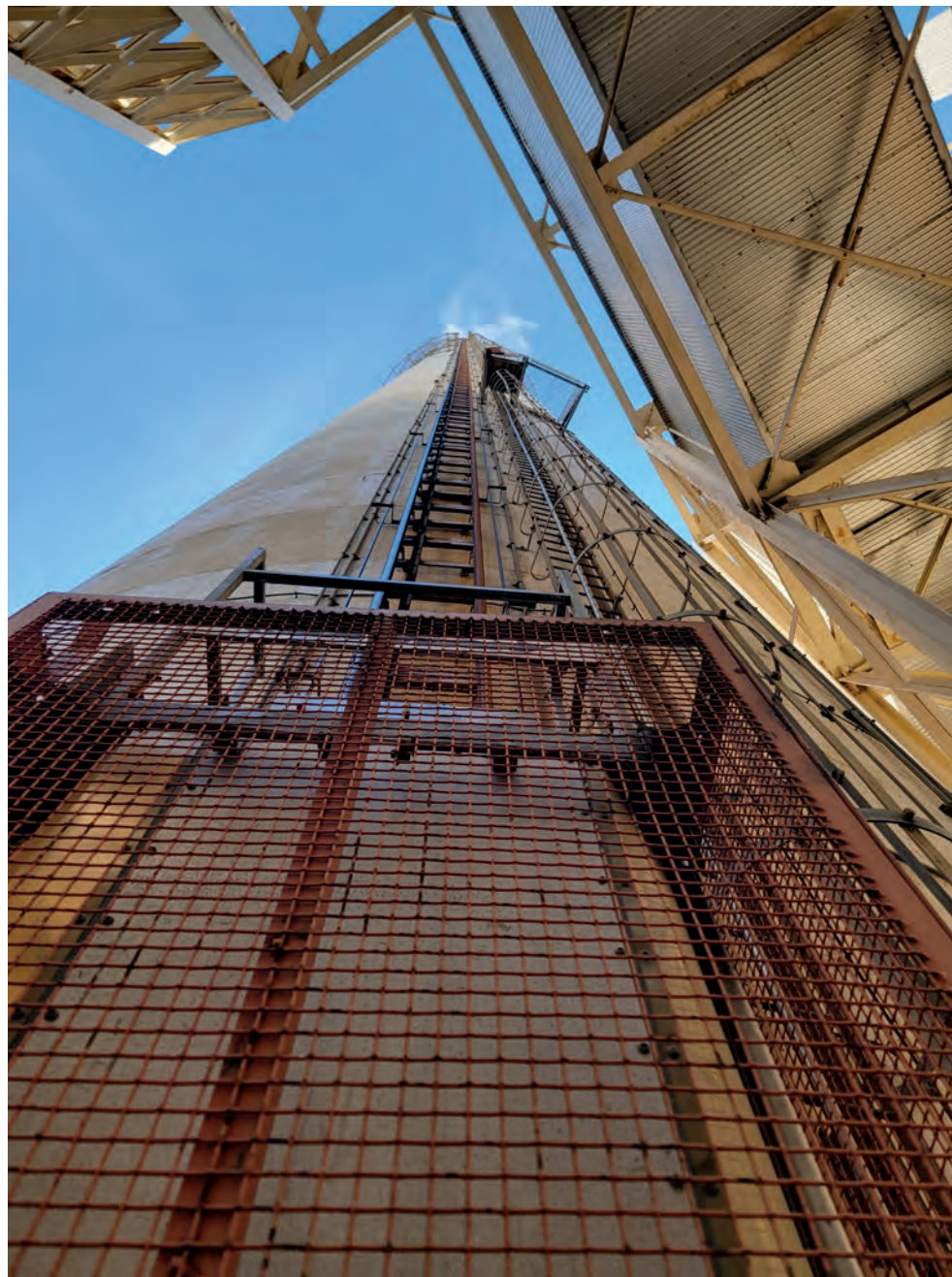
Rack-and-pinion stack elevator at a power generation plant
